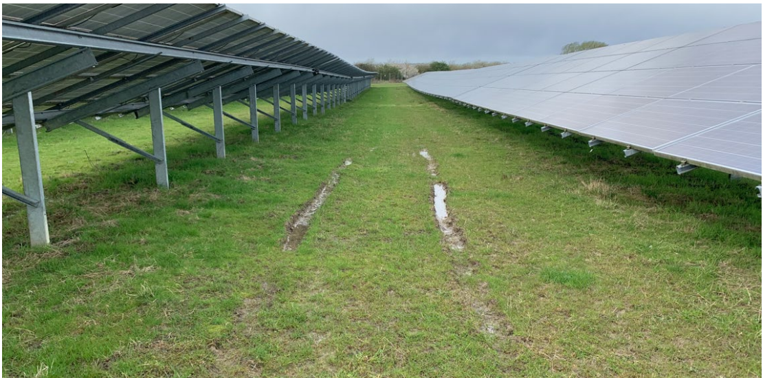
Photo 49: Ruts Caused by Vehicles
